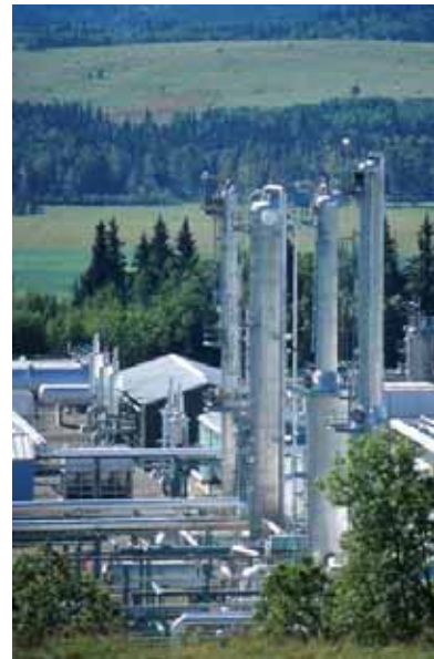
Gas power plant.
